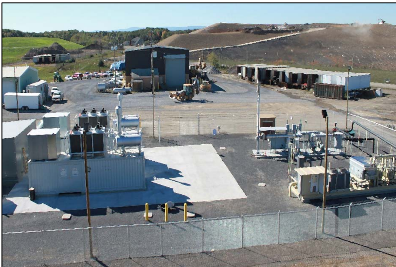
Landfill Gas to Energy Plant
